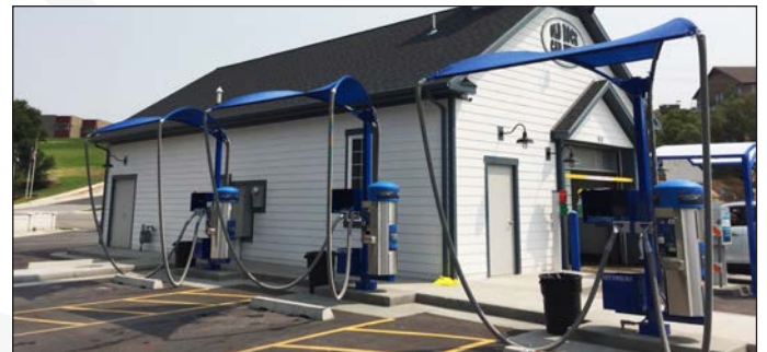
PICTURED: (3) Premier Single Express-2 Vac w/ Meter Box, Single Vac Station with Dual Boom, Canopy Add-on, Towel Bins, Blue Powder Coating.
